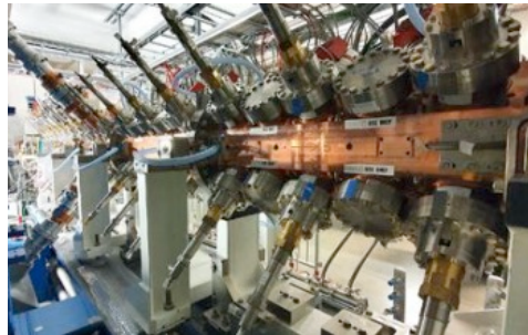
RFQ installed in the tunnel
