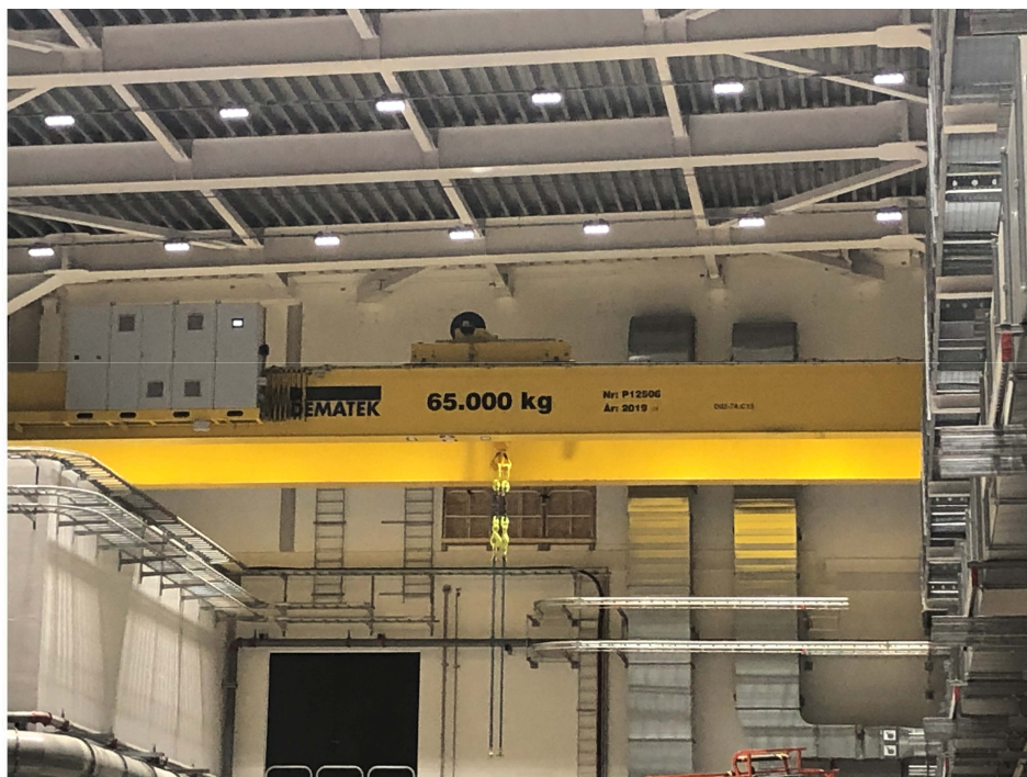
Figure 7.3: Largest existing ESS overhead crane currently in operation in the D02 Target building
